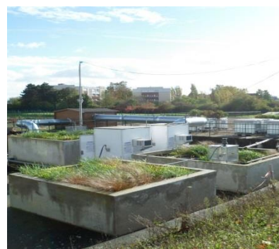
Fig.1 Overview of the experimental site with : the shelter receiving the extraction fan module, the pipe carrying the exhaust coming from tunnel, the biofilters fed from below with exhaust air and at the foreground the witness biofilter. On the two active biofilters the sampling chambers linked with the equipments measurements and in the background stand the water tanks used for the irrigation of the biofilters
