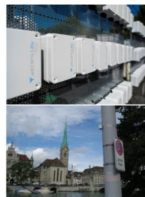
LP8 sensors at a rack at the air quality monitoring station in Duebendorf (top) and a single LP8 sensor deployed in the city of Zurich (bottom).
