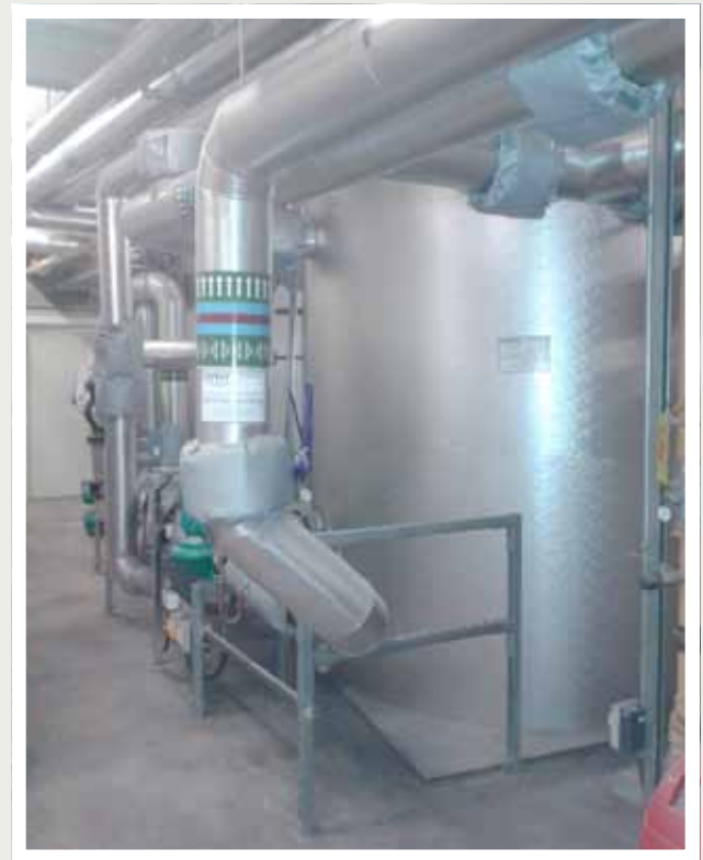
Figure 15. 'Fit and forget' – biomass boilers
