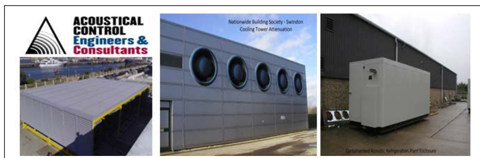
Figure 2: Weather Louvres, Cooling Tower Attenuation & Acoustic Refrigeration Plant Enclosure.
