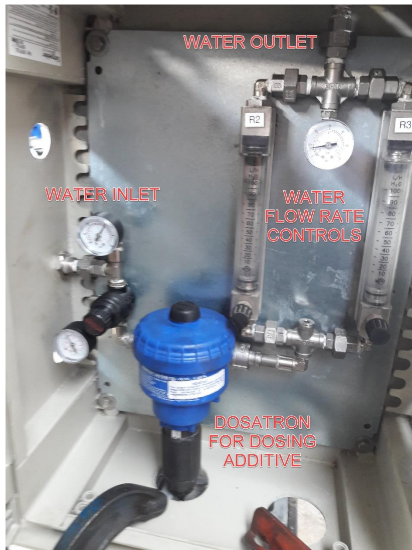
Figure 4-8 Water and additive control panel
