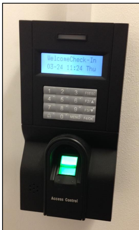
Figure 1 Redundant Access Control Reader at UH
