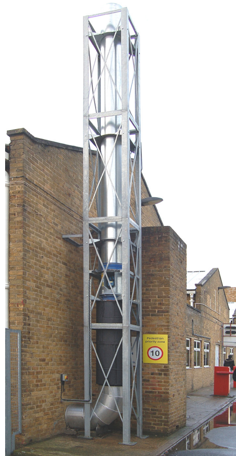
Figure 2. Ventilation system exhaust stack. The lower two metres (up to the fan) have sound-reduction cladding; discharge is approximately 8.5 metres above ground level.
