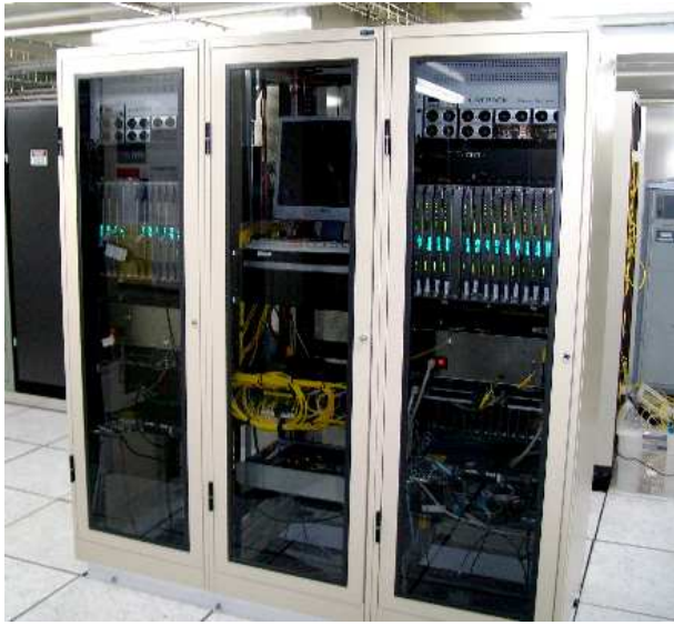
Figure 14. The CABB rack as installed in the fully shielded ATCA correlator room.
